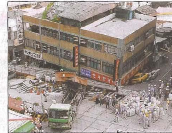
The foundations of this four-storey building give way in the aftermath of the MRT cave-in.
